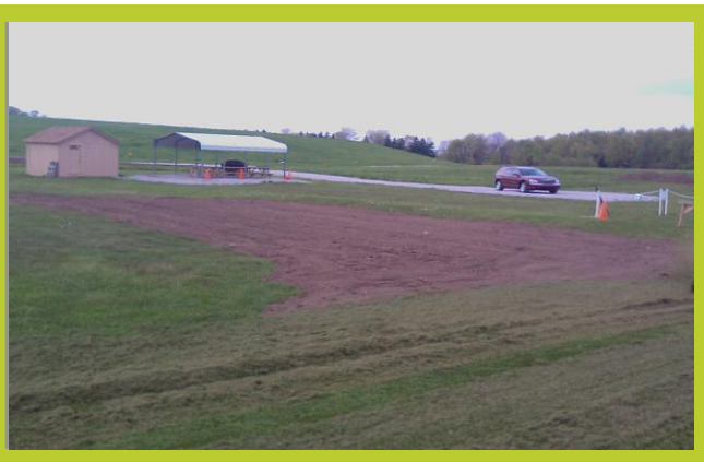
Here you see the large swale that was filled in at the south end of the pits. The swamp on the north end of the runway was also filled.
